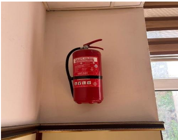
7. Fire Hidrant (Baku State University, Azerbaijan)
