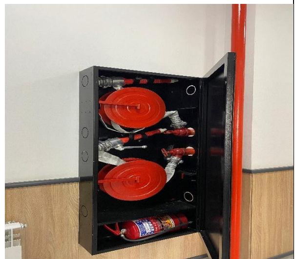
4. Fire extinguisher cabinets all over the campus (inside)
