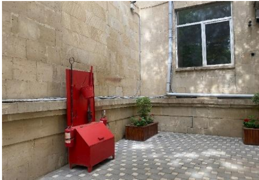
5. Fire extinguisher cabinets all over the campus (outside)
