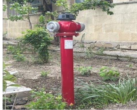
6. Fire Hidrants in the yards
